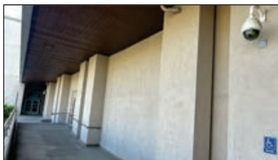
Figure 70 - PTZ Exterior Camera
