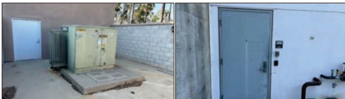
Figure 52 - Lack of Door/Opening Numbering displayed (RCC)
