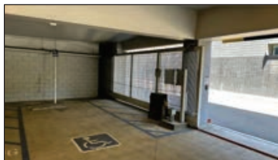
Figure 179 - Parking Garage Gates (District Office)
