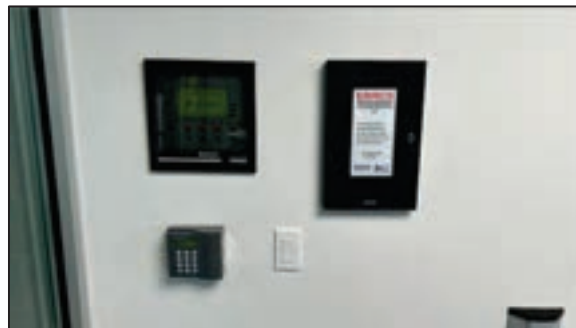
Figure 85 - Emergency Responder Radio Communication System (ERRCS) panel at the Building of Business and Law, RCC
