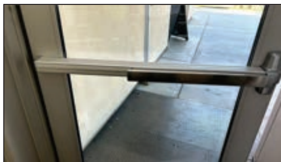
Figure 84 - Electrified panic bar with no dogging – SAS Building (MVC)
