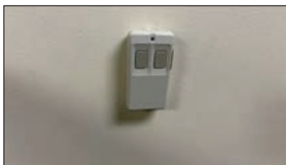
Figure 63 - Wireless Lockdown Button RCC
