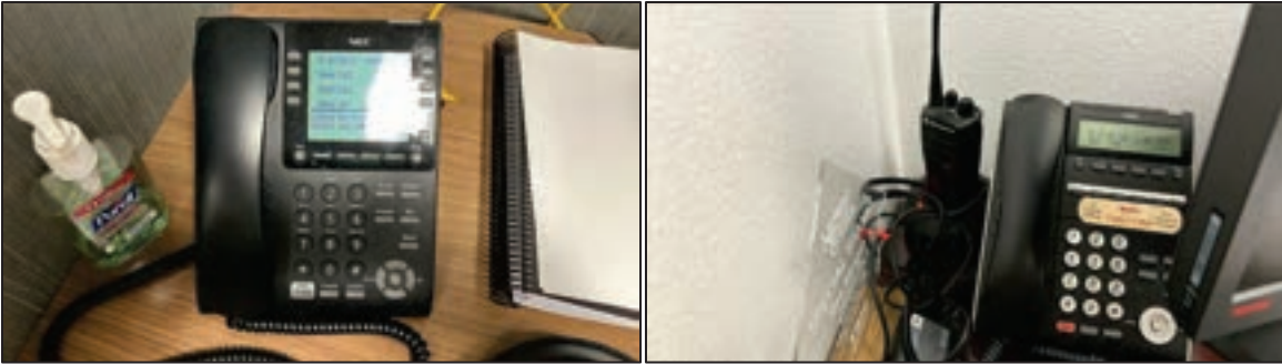
Figure 386 - NEC VoIP Telephone Handsets (New and Old)
